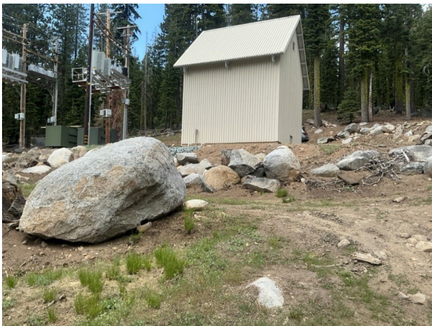
Figure 4.9.1.2-1: Cabbage Patch Switchyard and Substation
