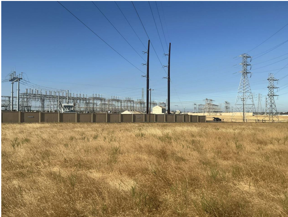
Figure 4.9.1.1-1: View of the Bellota Switchyard and Substation
