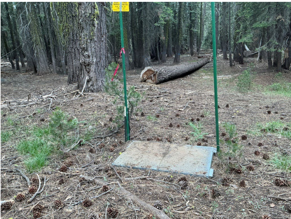
Figure 4.9.1.2-3: View of an Electric Vault on Off-road Section
