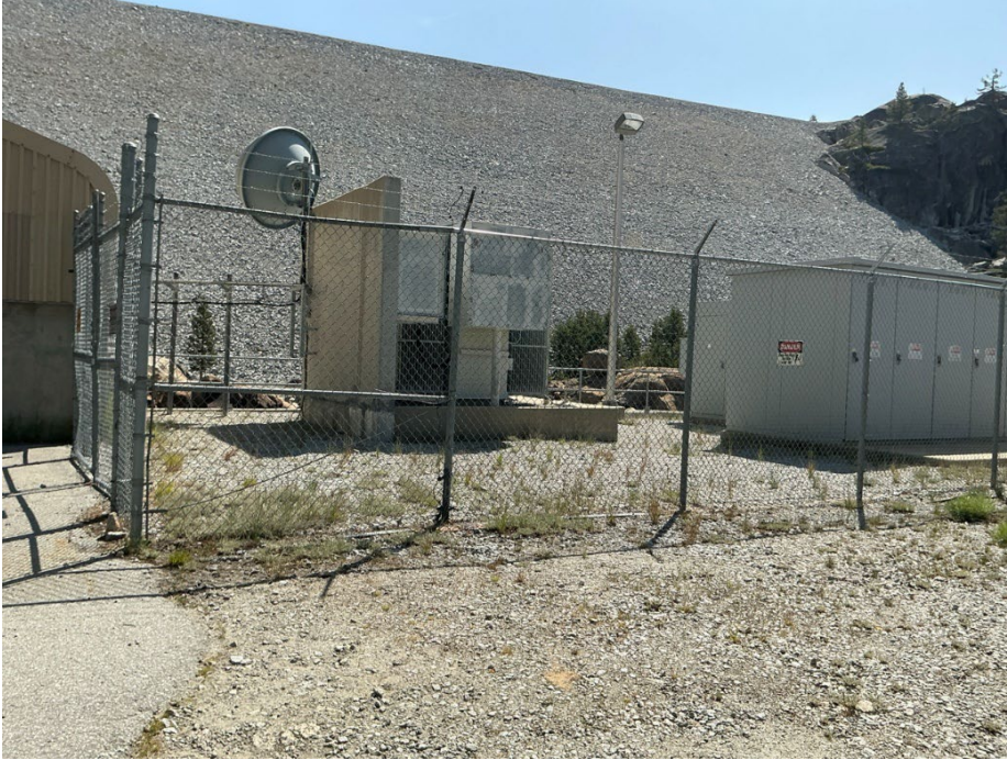
Figure 4.9.1.2-4: Spicer Meadow Powerhouse Switchyard (Dam in Background)
